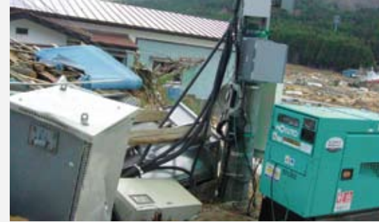
A generator installed at a base station.
