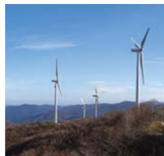
Wind Farm Hamada
