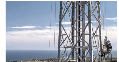
Mobile phone base station
